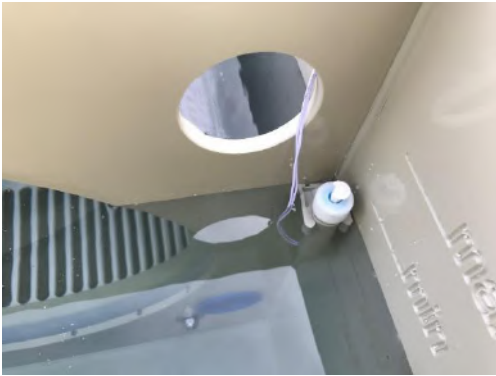
Float is in 'normal' position, pond pump is on
